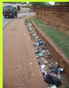
Waste blocking a storm drain. Bamako, Mali
